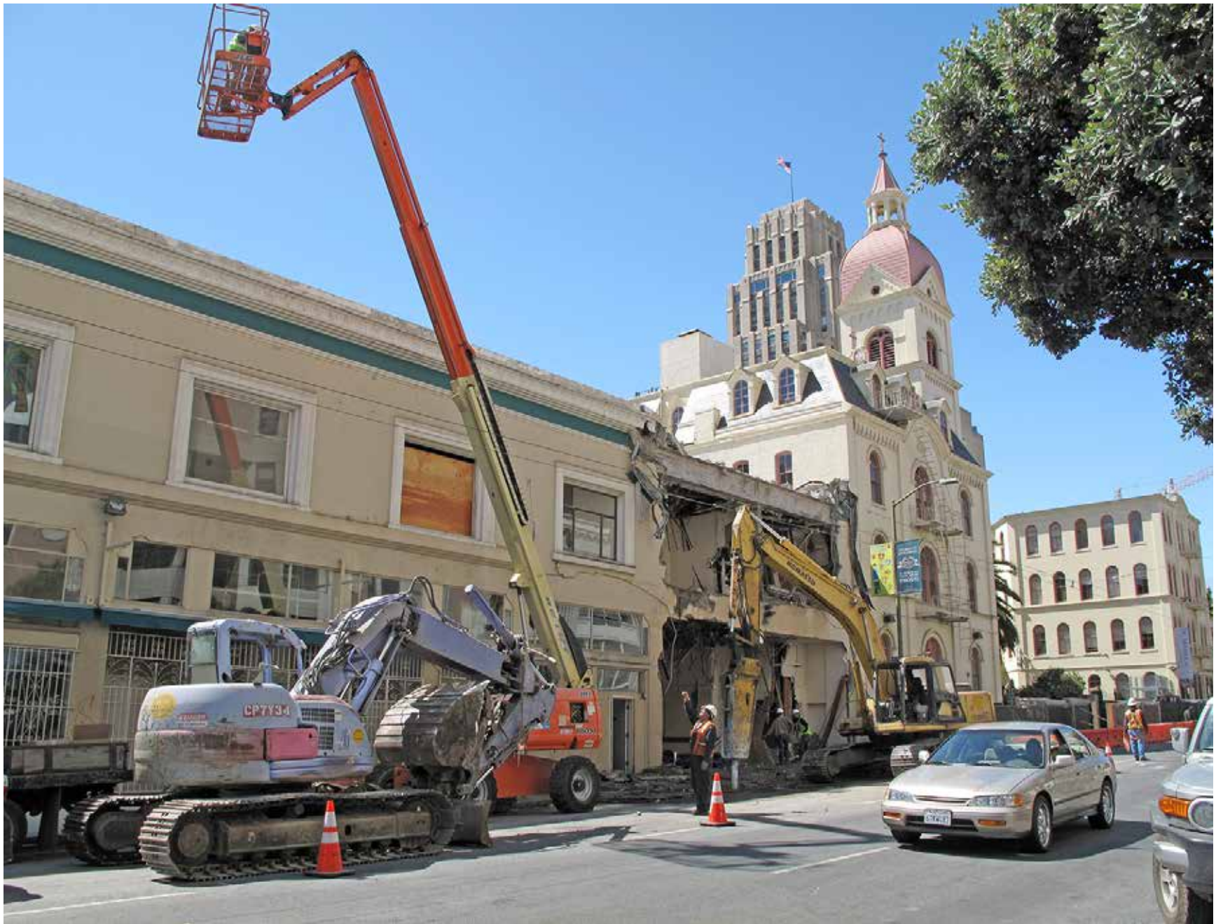
Demolishing the landmark St. Anthony Foundation offices and Dining Room buildings began Sept. 4. Next door is St. Boniface Church with De Marillac Academy at right.
