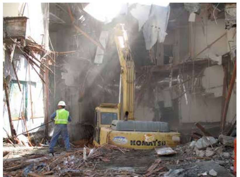
A ghostly cloud of dust rises from falling plaster and concrete, but a steady stream of water controls the air-borne particles.
